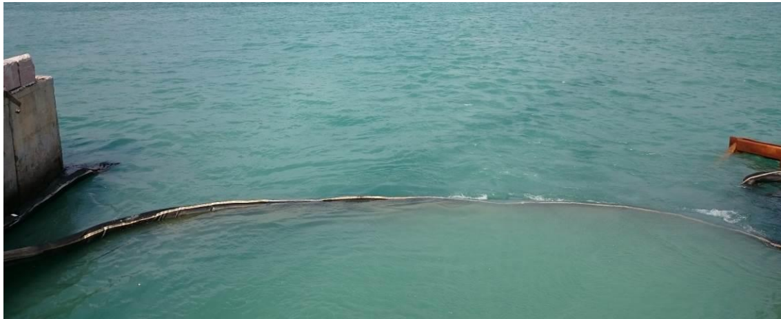
Photo of Silt Curtain for Culvert Channel for Final Stage of Works
